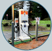
Electric Vehicle Infrastructure
